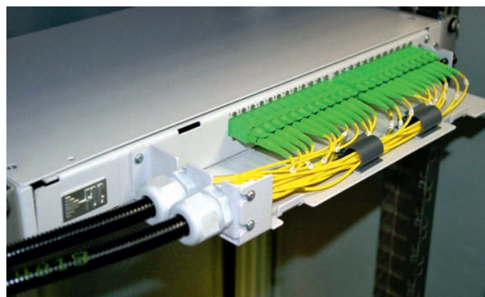
Figure 4 OKE (splice box) with optimized cable management
