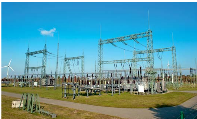
Bertikow substation (source: 50Hertz)
